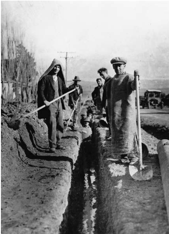
Above: Albert Malam (far left) and others ditch-digging in 1932. Tasks such as this typified Depression-age relief work, partly driven by concerns that work schemes should not compete unfairly with the private sector. (Photographer unidentified, Alexander Turnbull Library, F-27086-1/2)
